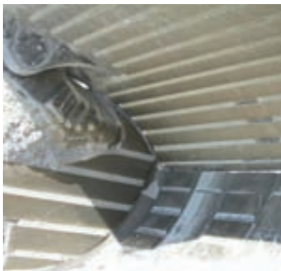
Minimal wear has occurred during the test program retaining the integrity of the bucket operation. Small grooving in the structural base of the bucket can be seen
